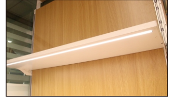
The installation is complete.
